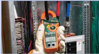
Collecting current measurements and associating them with the right component identified on an infrared image, can be a complicated and cumbersome process
